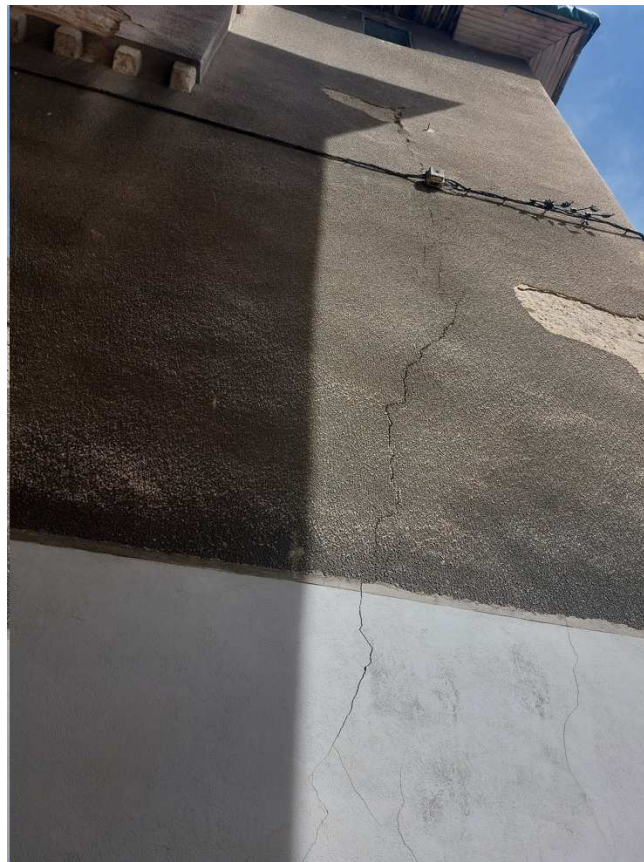
Figure 1: Fissure verticale en façade.
